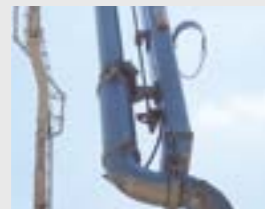
Shut Off valve on endhose
