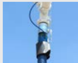
Shut Off valve in pipeline
